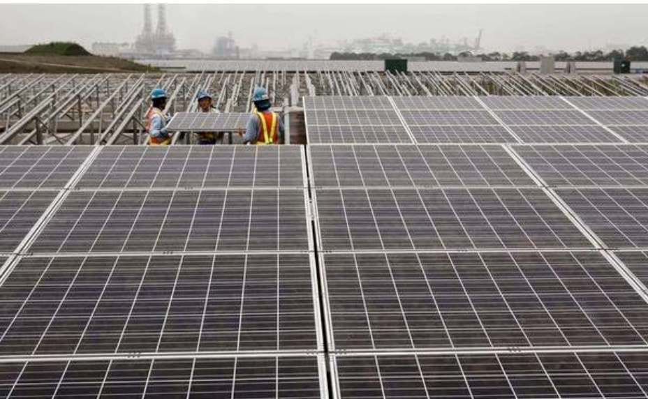
Solaranlage in Monarchak
