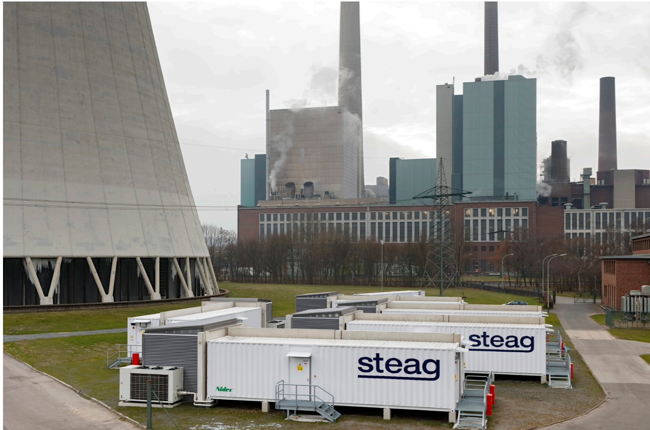
Realised 15 MW system at Luenen power plant site © STEAG
