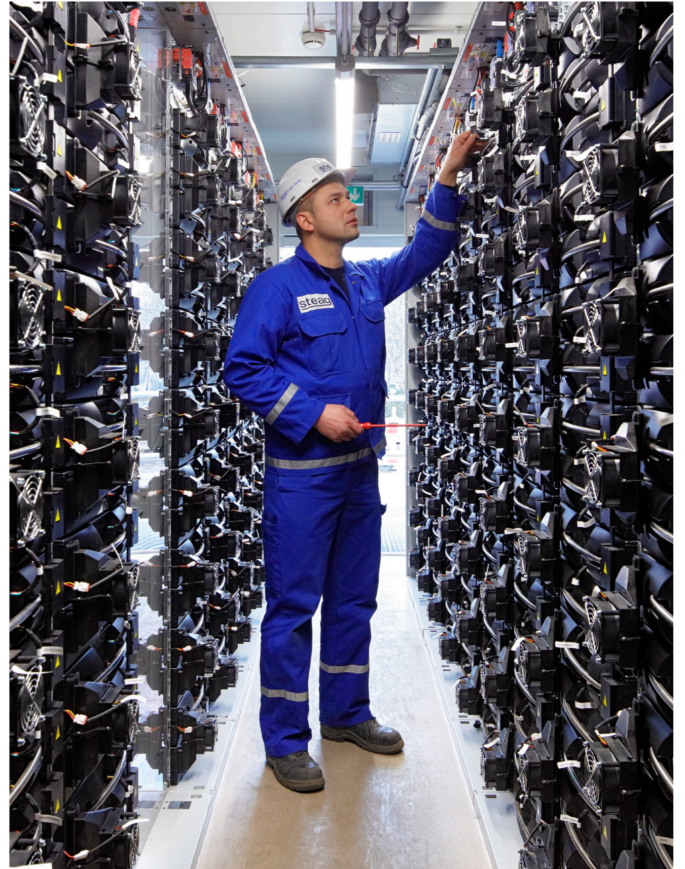
Inside the battery container © STEAG
