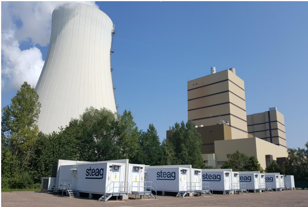
Picture 1: STEAG's large scale battery system at Völklingen-Fenne site
