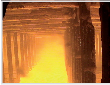
Fig. 5. Left: Unit D: Supporting tube bulkhead after being cleaned by a steam blower (Source: EUvis insitu).
