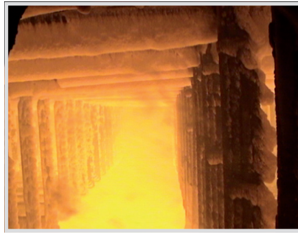
Fig. 6. Left: Unit D: Supporting tube bulkhead cleaned six hours ago (Source: EUvis insitu).
