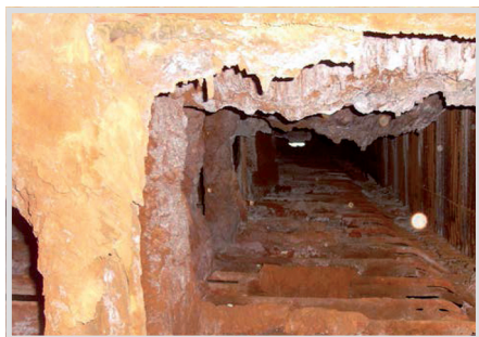
Fig. 1. Unit A: Fouled supporting tube bulkhead.
